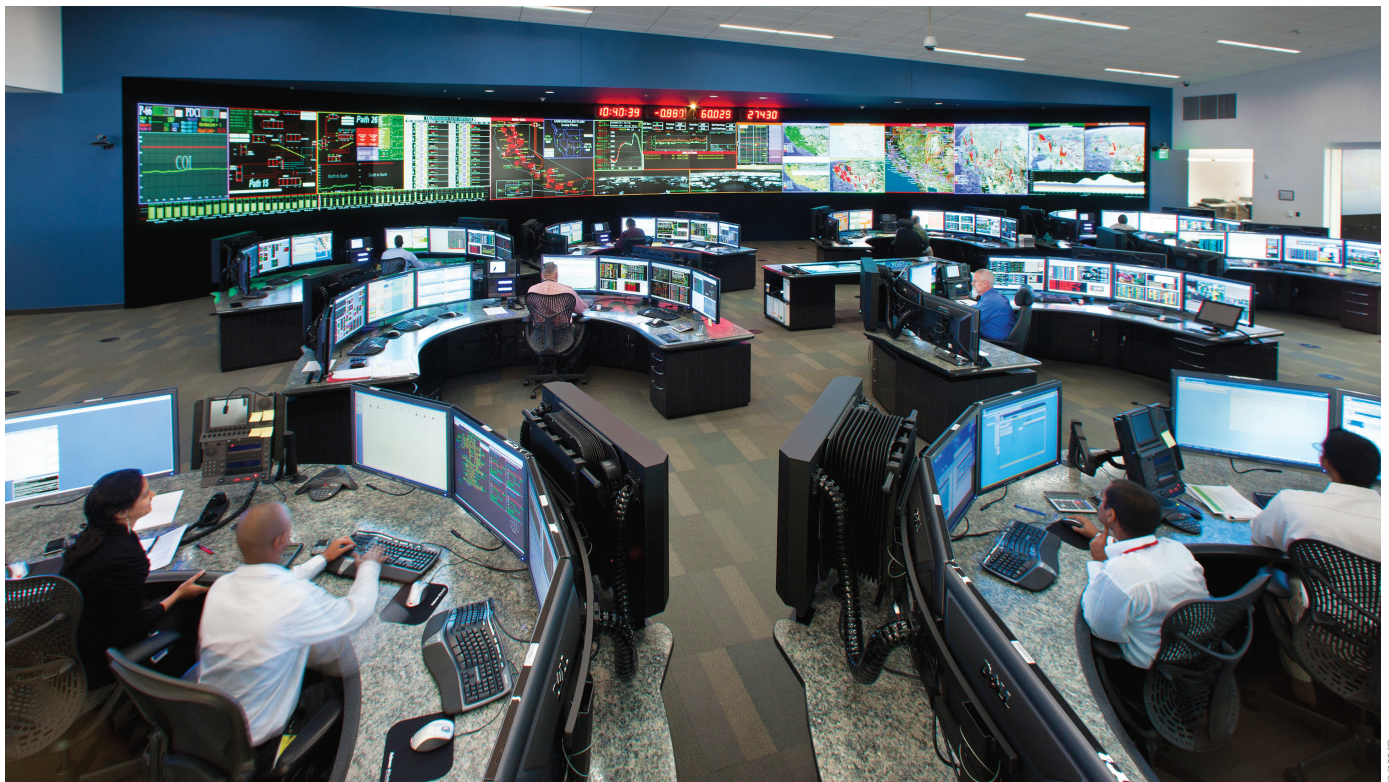
At the California Independent System Operator (CAISO) grid control center, electricity supply and demand are constantly balanced to maintain reliability.
