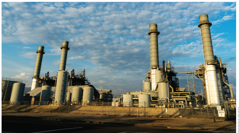
Southern California Edison’s Mountainview Generating Station is one of the nearly 200 grid-connected natural gas power plants in California.
