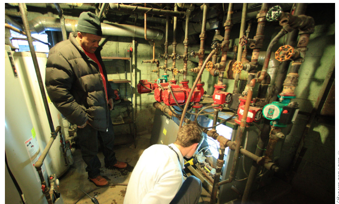
An efficiency specialist examines the systems at a multifamily building to identify cost-effective energy-saving measures. A CPP compliance plan that prioritizes efficiency efforts such as this can benefit all Michigan residents.
