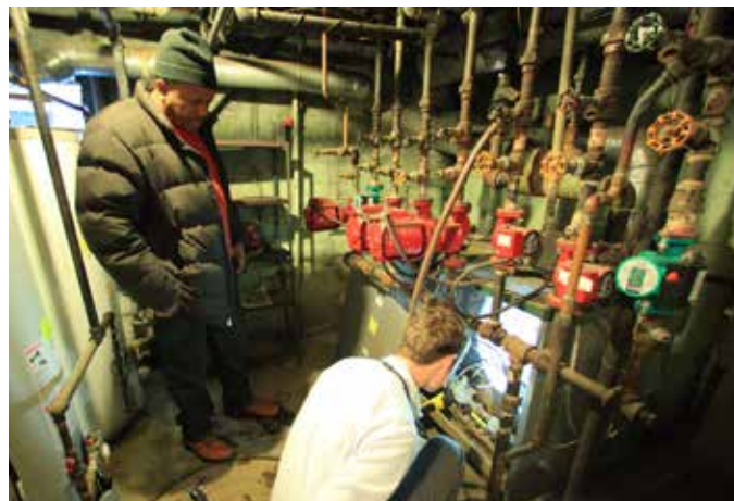
An analyst from Elevate Energy examines the systems at a multifamily building in Chicago to identify cost-effective energy-saving measures. A CPP compliance plan that prioritizes efficiency efforts such as this can benefit all Illinois residents.
