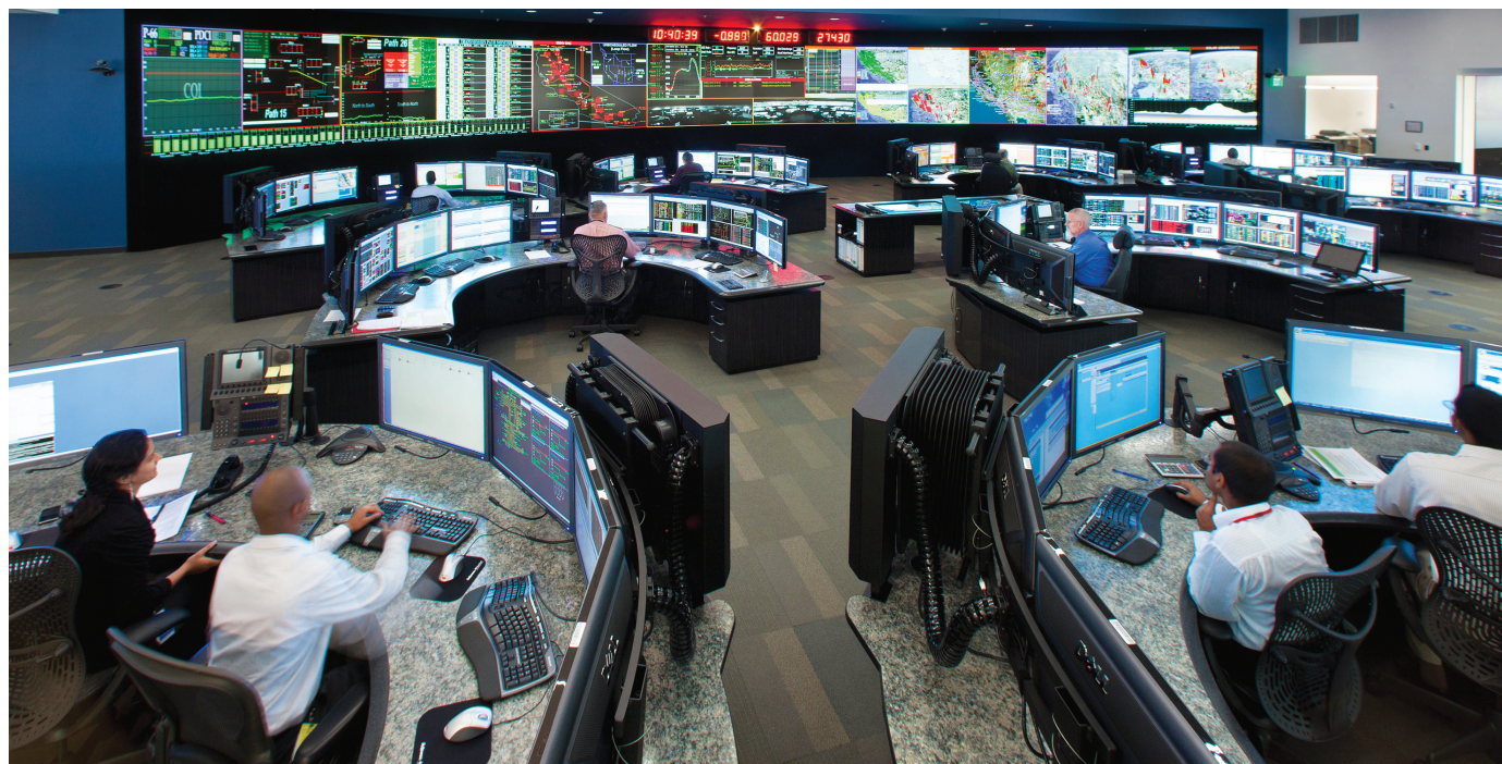
At the California Independent System Operator (CAISO) grid operation control center, electricity supply and demand are constantly balanced to maintain reliability.
