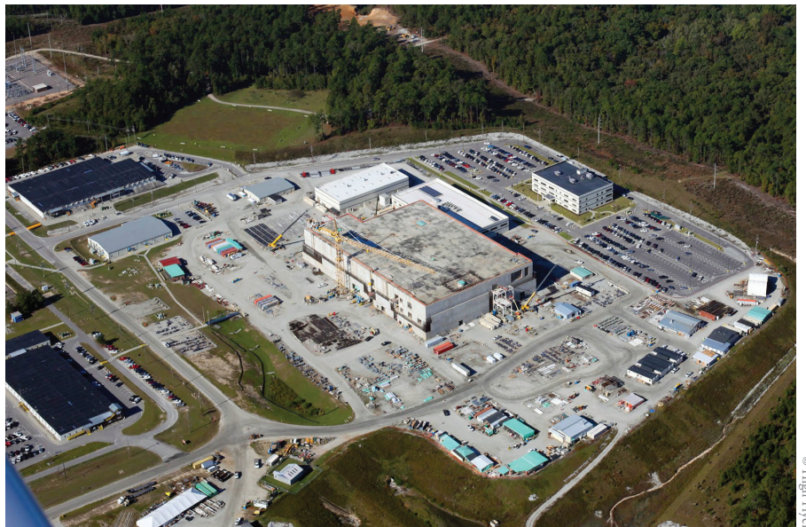
Construction of the MOX Fuel Fabrication Plant at the Savannah River Site, years behind schedule and billions over budget, remains unfinished.
