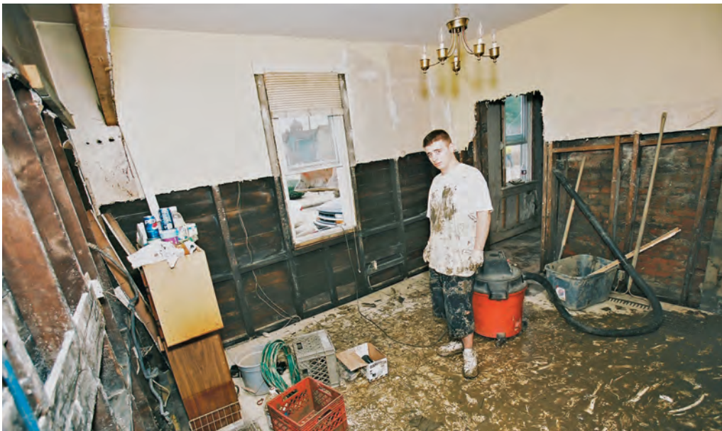
After a 2004 flash flood inundated this home in Bridgeville, PA, all of its baseboards and insulation were removed to prevent mold and mildew. Long after a flood's waters have receded, residents often continue to struggle with mold-induced respiratory illnesses, depression, and the stress of repairing or rebuilding an uninhabitable home.
