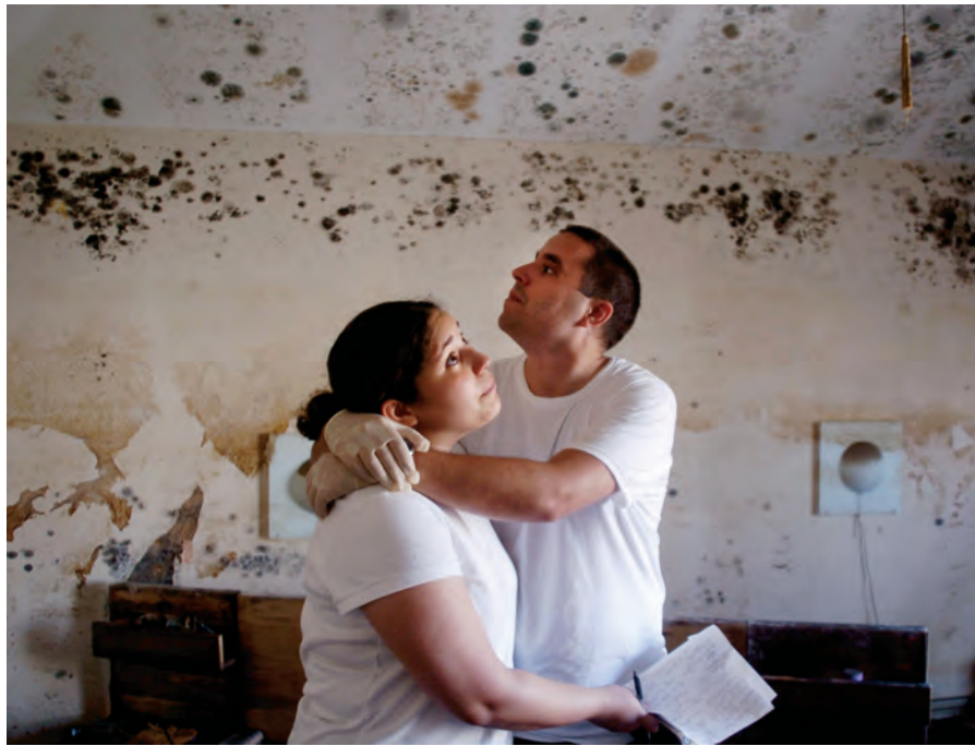
A couple stands in despair in the mold-infested bedroom of their first home, which they had finished remodeling shortly before it was flooded by Hurricanes Katrina and Rita. In the aftermath of the storms, an estimated 46 percent of homes in New Orleans and surrounding parishes had some mold contamination and 17 percent had heavy mold contamination (Barbeau et al. 2010). Inhaling the spores from mold can trigger allergic reactions and exacerbate asthma.
