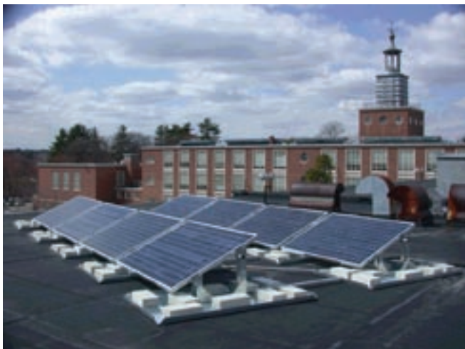
Wellesley, MA High School solar photovoltaic array. Courtesy of Schott Applied Power.
