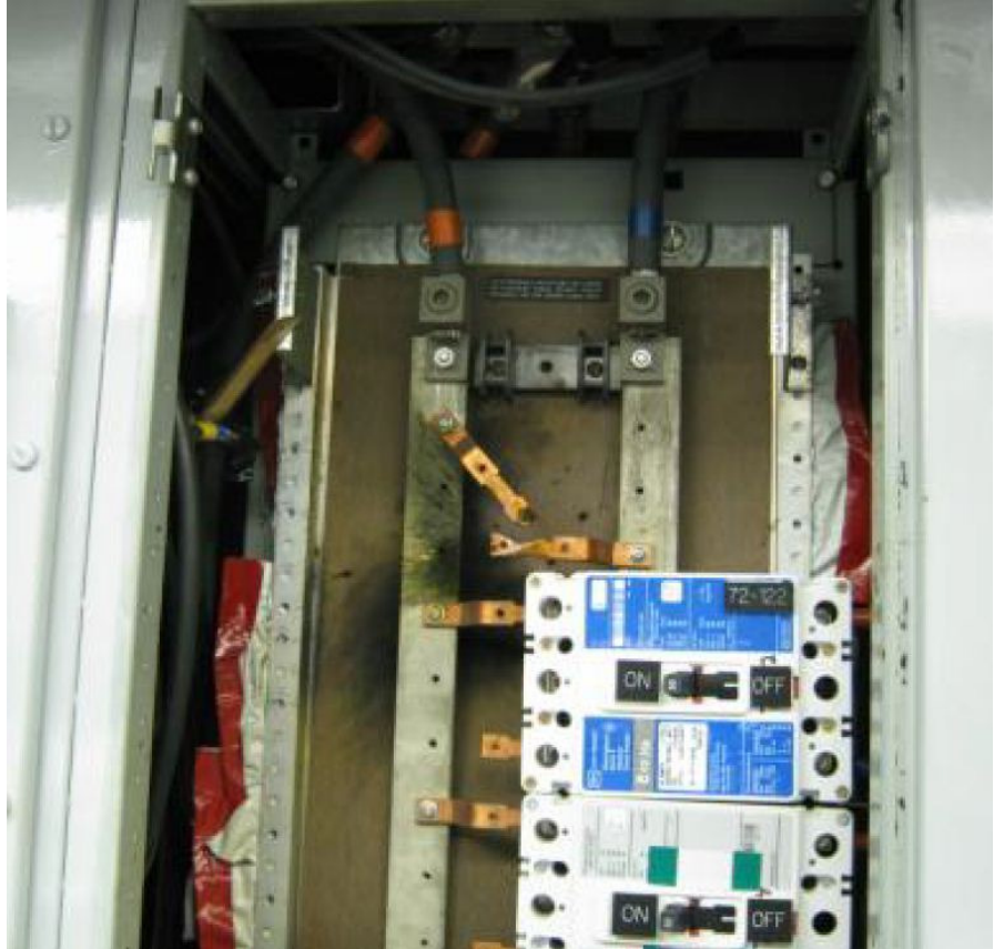
The distribution panel at Palisades where the disruption in electrical power started. Source: NRC.
