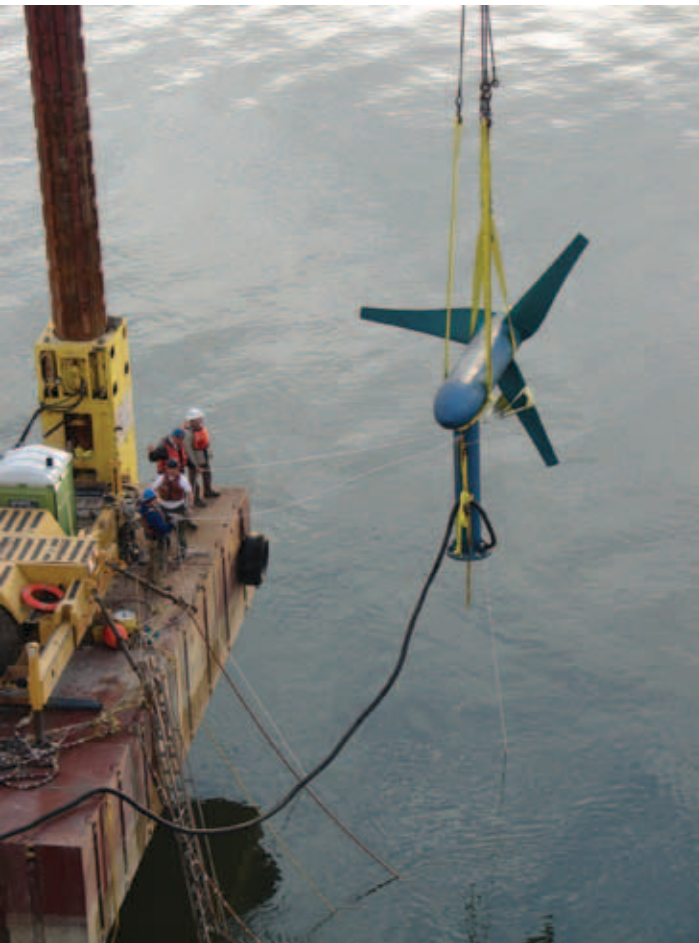
A tidal turbine in New York City's East River.
