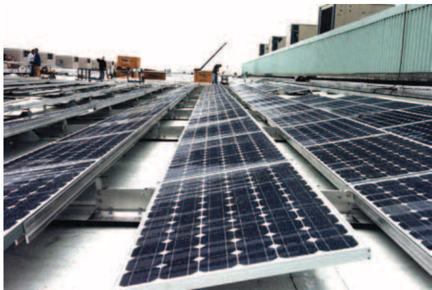
New Jersey policies promoting clean energy helped finance the nation's largest single-roof solar project (at the Atlantic City Convention Center). Unveiled in March 2009, the project meets 26 percent of the building's electrical needs and avoids the release of more than 2,300 tons of CO 2 annually.
