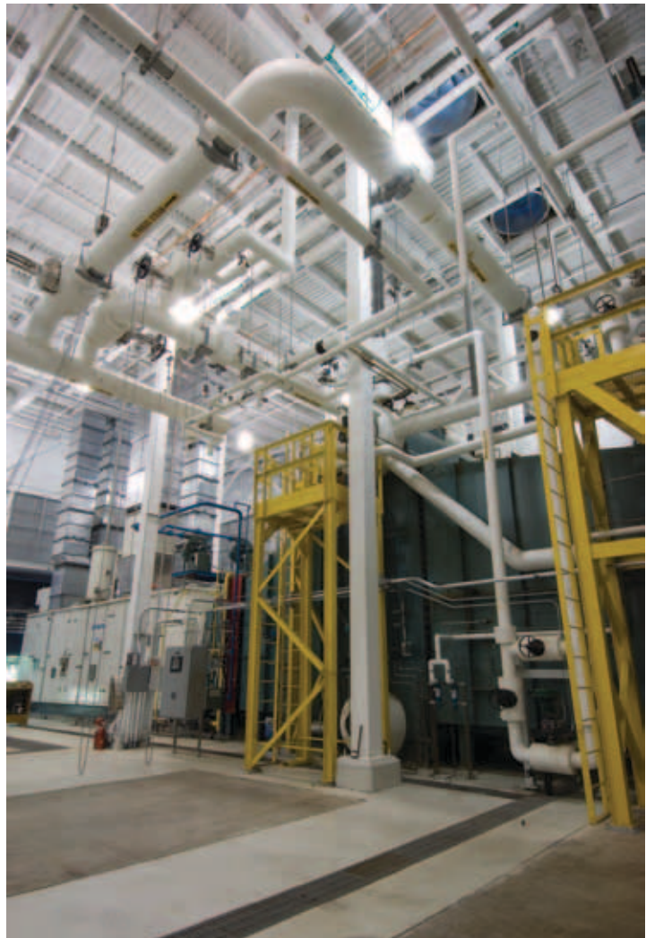
A combined-heat-and-power plant at the University of New Hampshire provides heating, cooling, and electricity to the majority of buildings on the main campus while reducing carbon emissions and saving money.
