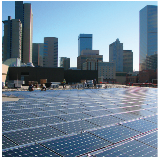
This 300 kW solar PV system atop the Colorado Convention Center in Denver is one of the largest rooftop solar systems in the state. Smaller residential rooftop PV systems have also become popular as costs have declined and innovative financing mechanisms have been developed to help meet the demand created by Colorado's RES.
