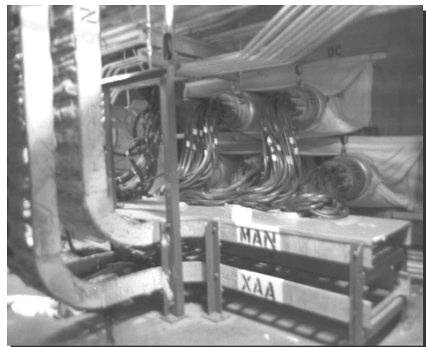
Power cables run through trays, conduits and tunnels, impeding the ability to inspect them, and to detect and suppress fires.
